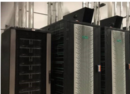
FIGURE 2. Interior of a MDC
